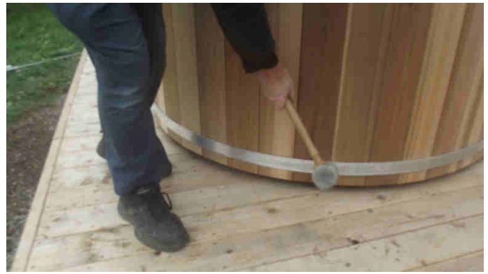
Figure 9.1 Hitting staves directly on the strap.
